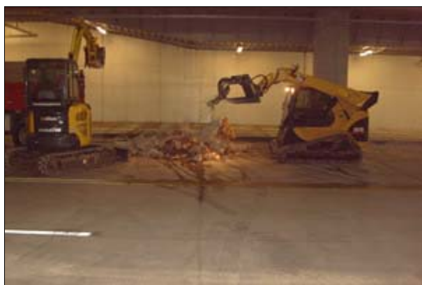
Earth and material moving equipment operating at the exercise helped organizers simulate the sights and sounds of an actual disaster response in progress. (Photo courtesy of Jim Remington)
